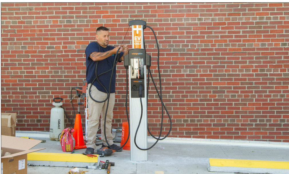
The EV charging station was installed by Plugshare, which is based in Albany, New York.
